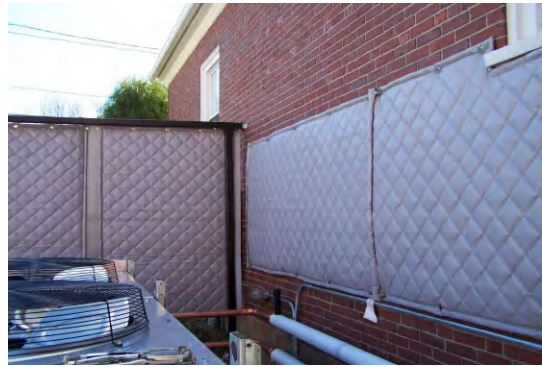
Generator noise control
